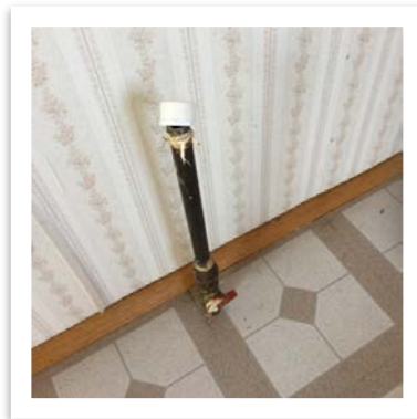
Incorrect type of gas line cap.
