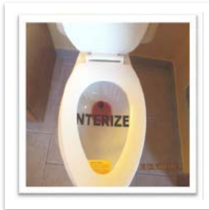
Properly cleaned and winterized toilet.
