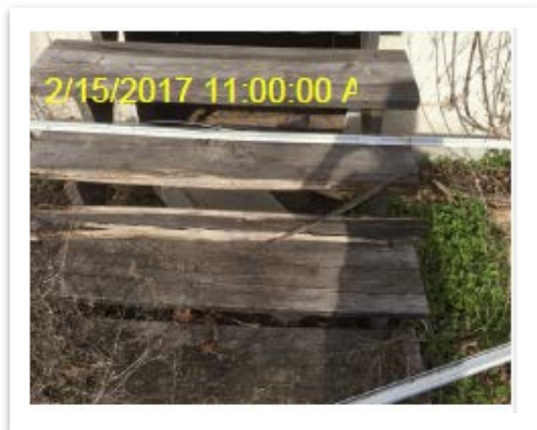
Damaged treads and risers.
