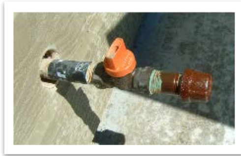
Gas line shut off and capped correctly.
