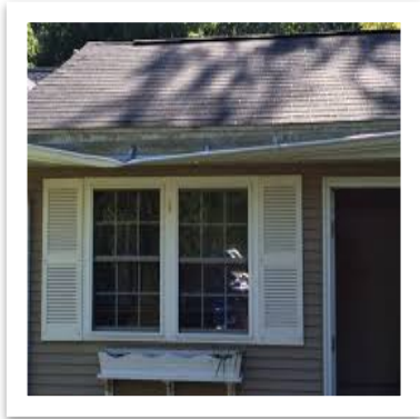
Section of gutter needs repair.
